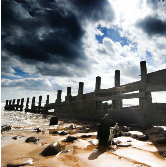
Dilapidated sea defence assets at Amroth Beach, Pembrokeshire
